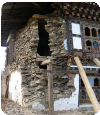
Figure 1. Damage pattern of stone masonry houses due to earthquake in Bhutan. The failure shows in-plane, out-of-plane and missing the key components like cornerstones and bonding stones.
