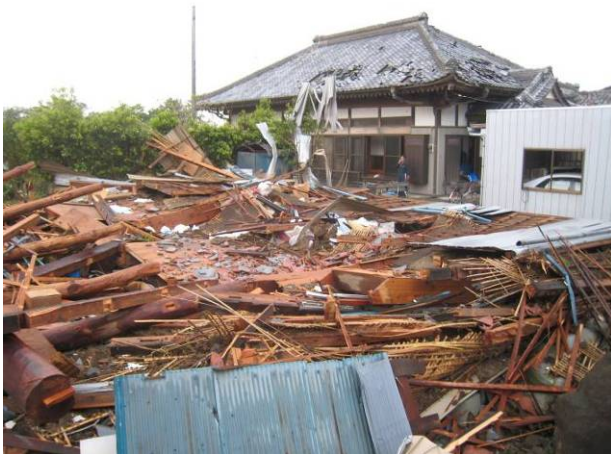
Photo 3 Wooden building B (this side, collapsed one)
