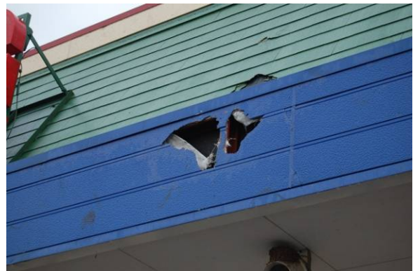
Photo 26 Evidence of collision to exterior material
