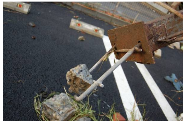
Photo 20 Pull out of column base shown in Photo 19
