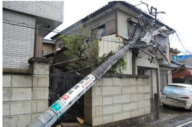
Photo 34 Broken / inclined electricity poles 2
