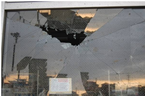
Photo 25 Evidence of collision to window
