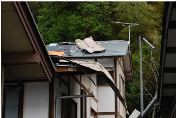
Photo 27 Scattered long steel roofing materials
