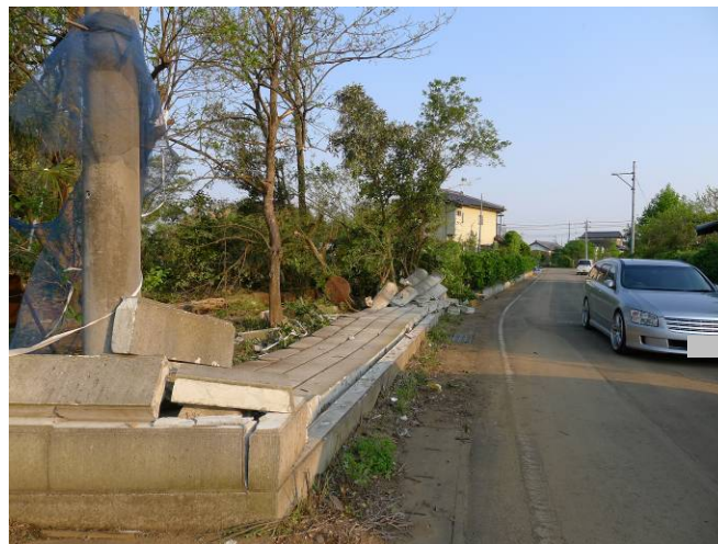
Photo 32 Collapse of stone fence
